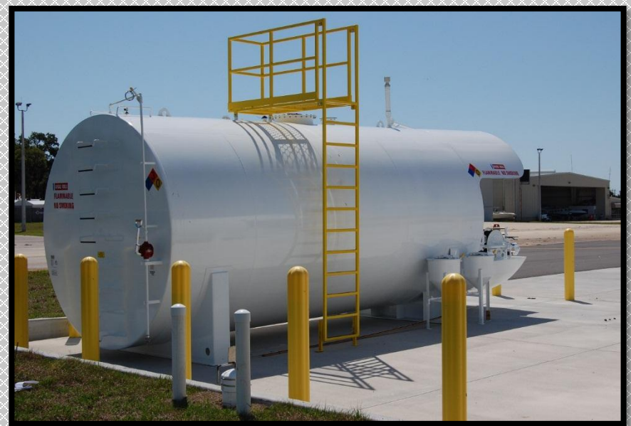
Fuel Storage Tank
